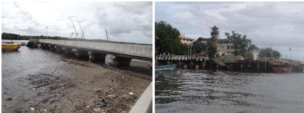
Plate 3-6: Shows Matondoni and Mangrove (KMA) jetties within Matondoni and Lamu Old town respectively
