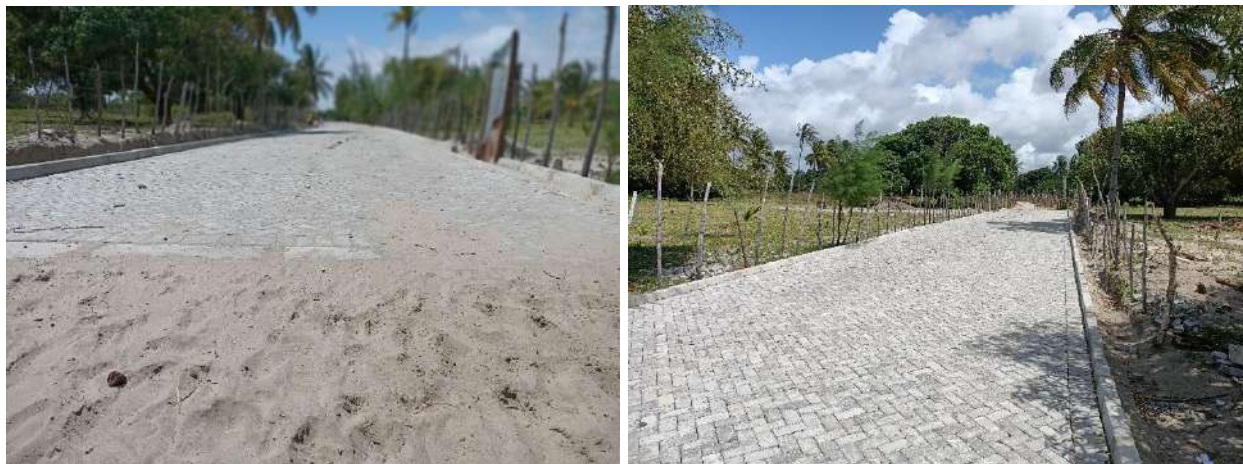
Plate 3-8: Cabro road under construction through the NCDF and KeRRA to connect Lamu and Matondoni settlements
