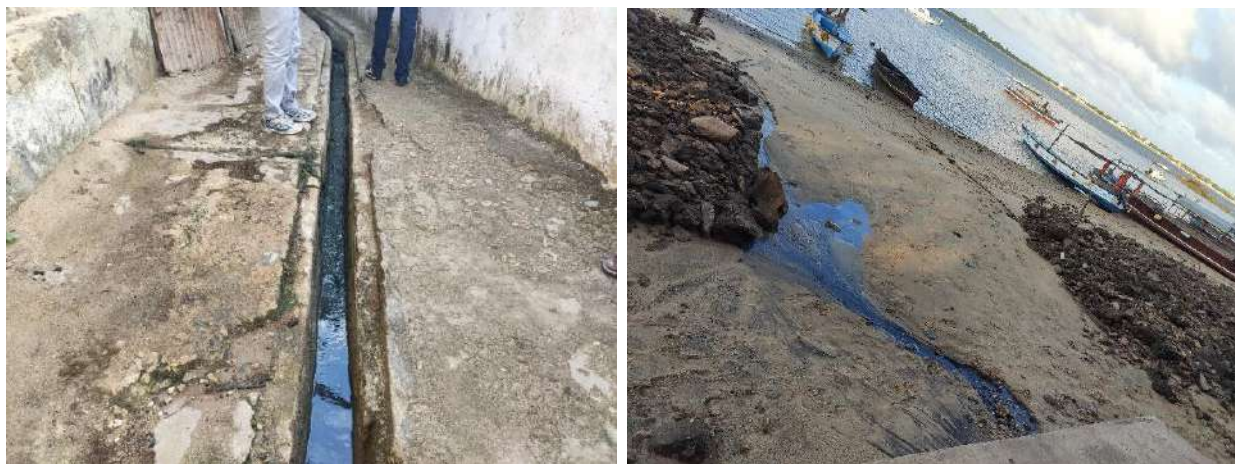
Plate 3-15: Shows an open drainage channel that empties into the ocean in Lamu town
