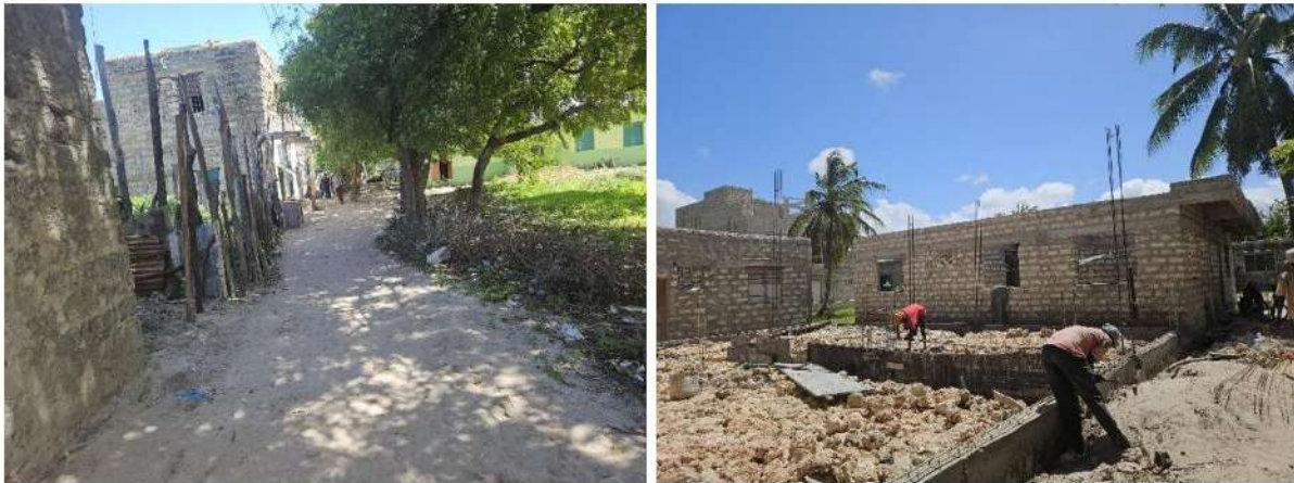
Plate 5-5: Irregular Street Layout; Residential Buildings under Construction in Areas with Tenure Insecurity
