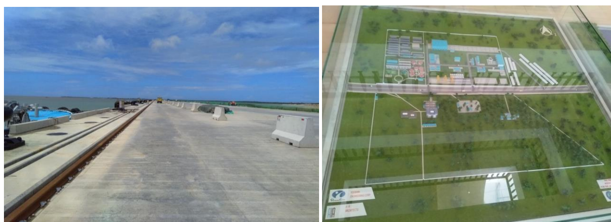
Plate 4-1: Left - Ongoing construction of berths; Right - Illustration Master plan for Lamu Port
